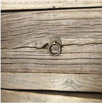
Small cracks along grain lines
