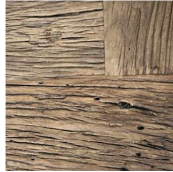
Small holes in wood
