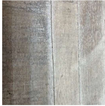
Small cracks due to seasonal temperature and humidity variations
